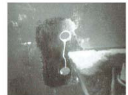
Photo of the crack in the database (The third line of the metropolitan expressway (Part 2))
