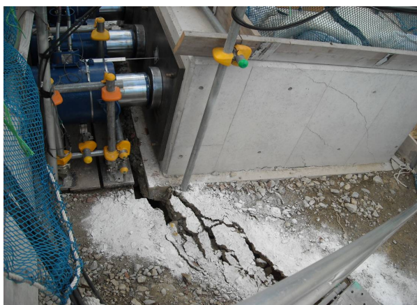
図-6 杭降伏時周面状況
