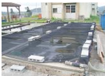
Fig.2 Sea water tank
