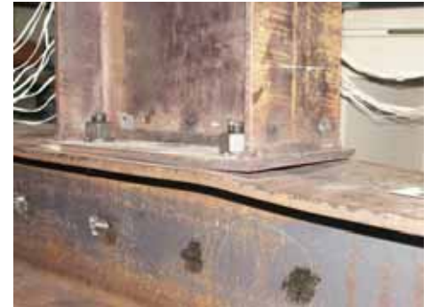
Fig. 5 Test specimen after loading (Test 3)
