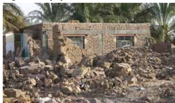
Fig. 3 Completely collapsed adobe house
