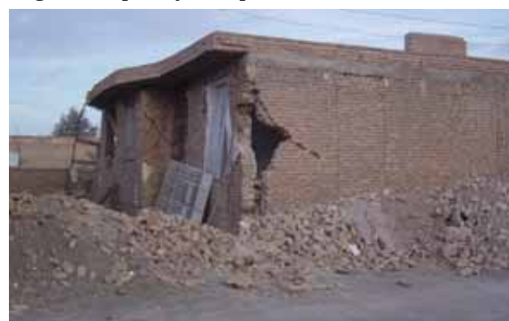
Fig. 4 Heavily damaged partially confined masonry house
