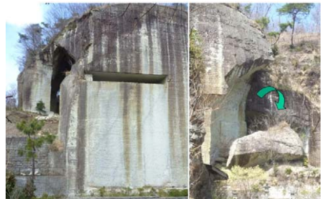
Figure 5. Partially collapsed semi-underground opening
