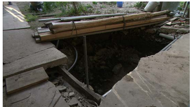
(a) A large sinkhole extending below the storage room and the main building
