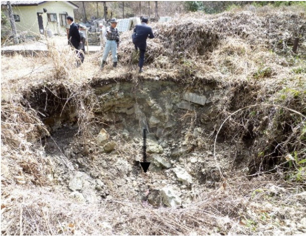
Figure 6. the settlement of back-filling material of the shaft
