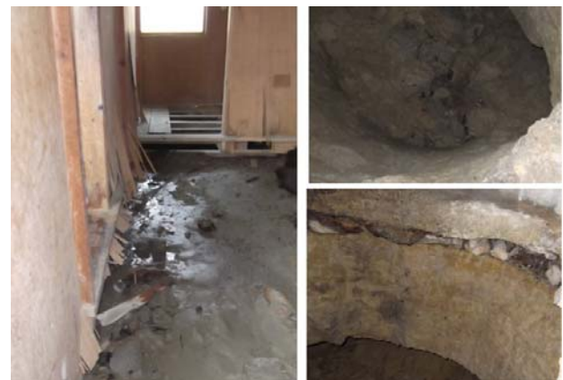
Figure 14: Some views of sinkholes in Wakayanagi town
