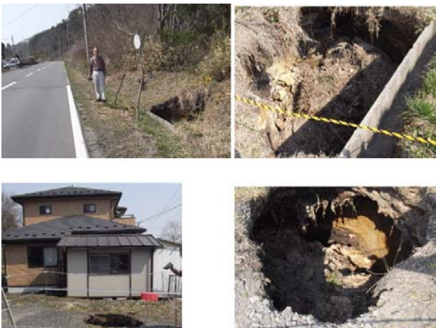
Figure 16. Views of sinkholes along a roadway and parking lot near Ohira Village
