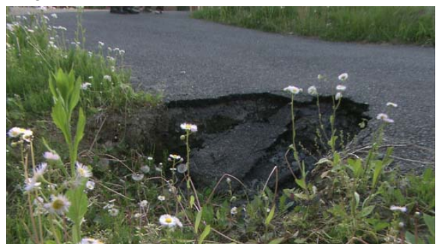
Figure 19. Sinkhole beneath the roadway in Ichinoseki (L3)
