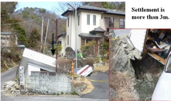
Figure 7. The settlement of back-filling material of the shaft and the fall of the hut and car into the shaft
