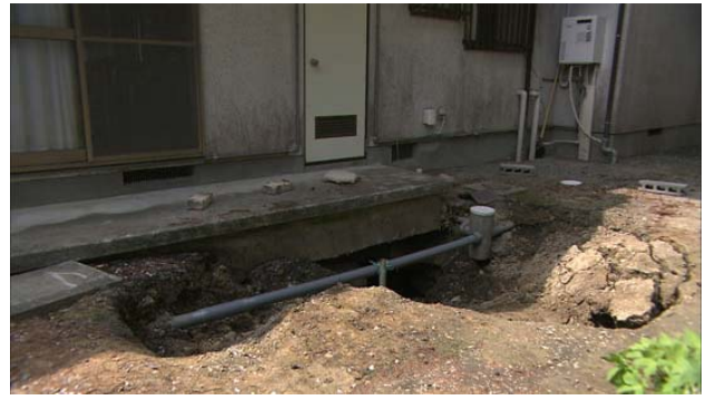
Figure 17: A sinkhole beneath a house in Ichinoseki. (L1). The size of the sinkhole enlarged after the April 7, 2011 aftershock.
