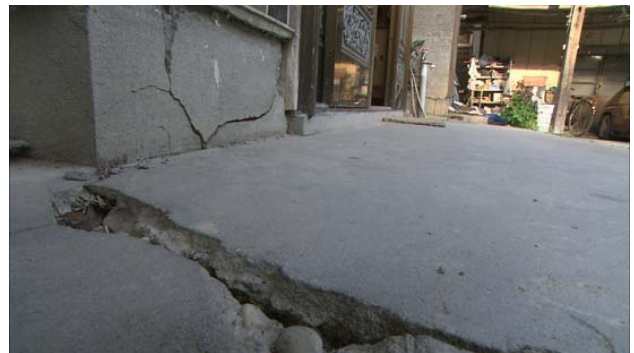
(b) Cracking of the concrete base and walls in the main building.
