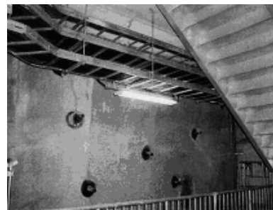
Photo 2 PS anchors in A powerhouse.
