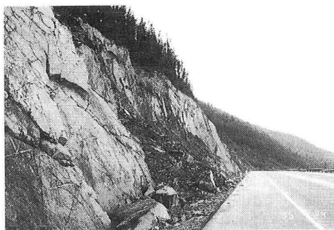
Photo 3 Curved sliding failure (P.3)
