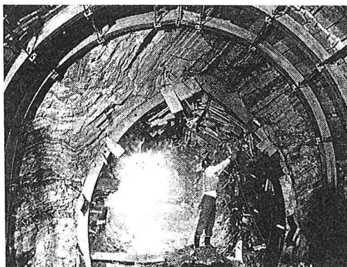
Fig. 2. Failure caused by kinking in tunnel.
