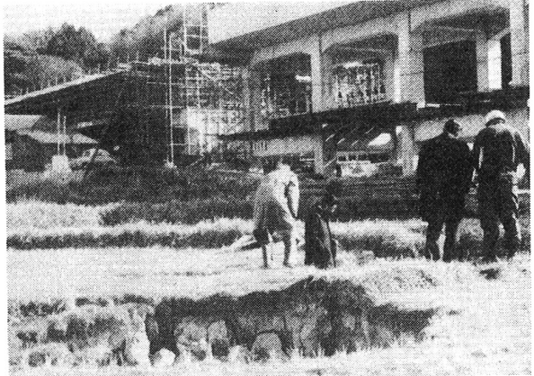
Photo.1 Cave-ins due to ground water drainage.
