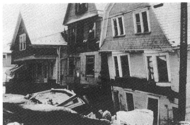
Photo.2 Home severely damaged by sinkhole in Pennsylvania.
