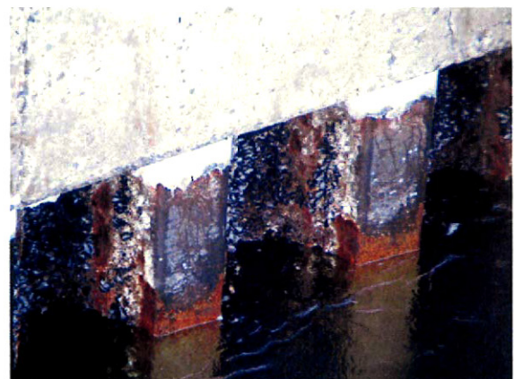
図-5 鋼矢板の流水接触痕
