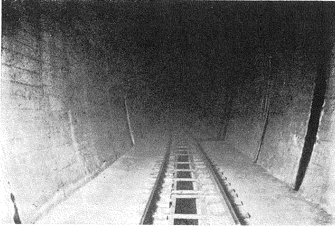
(2) 岩富隧道内のソリッドベッド、式道床 (2) Solid-bed floor in the Iwato-tomi tunnel.
