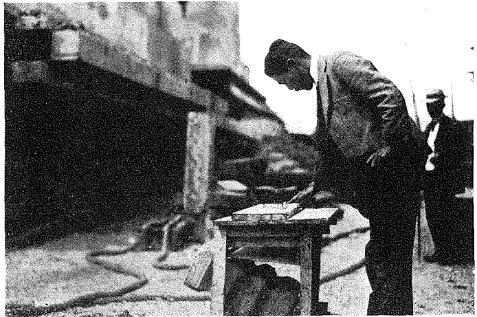
(6) Mr. Suyama, An Engineer In Charge, Is Just Now Going To Cut A Rope Off For Sinking Huge Concrete Caisson.
