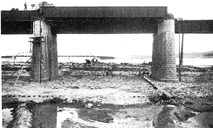
(8) View of Placing 60 Feet Girder after Raising the Piers 3 Feet with Concrete.
