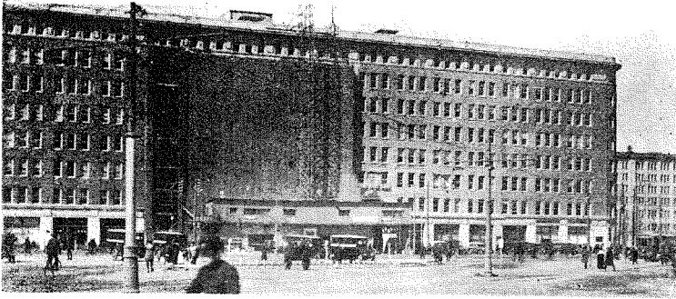
(4) View of Earth-Quake Proof Plastering on the Front Wall of "Maru Buil."
