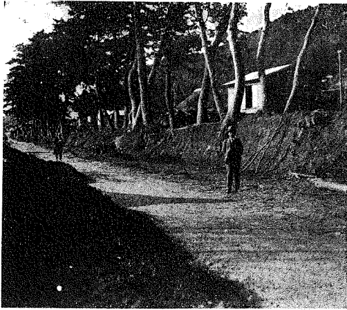
(7) 工事中の藤澤町宇車田松並木伐採前の景 (7) Road under Construction, Just Before Trees had been Cutting Down.
