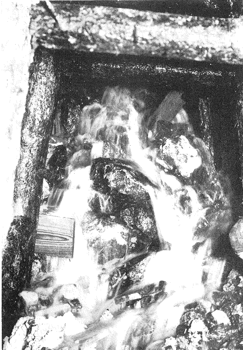
(10) A Gush of Water was Encountered at the Heading 200, from Tunnel Entrance.
