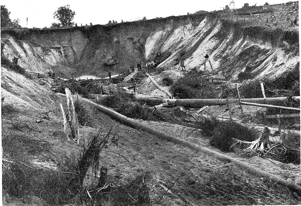
(5) The Pipe on Left Carries Sluiced Material to the Dam on Minimum Grade of 4%. The Other Two are Water Supply Pipes for the Giants.
