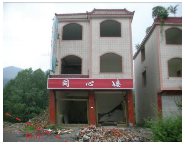
Figure 5-(b). The brick-concrete building was sheared to damage at the first floor near the rupture
