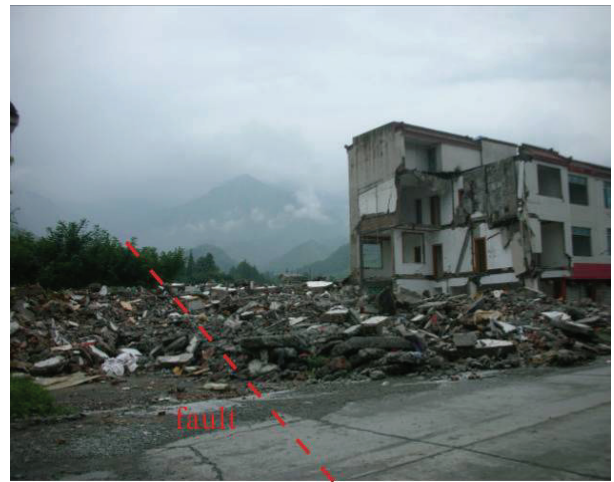
Figure 5-(a). The standing brick-concrete building near the rupture
