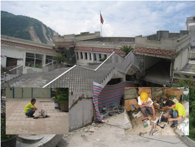
Figure7. Measuring points at the damaged school of Yingxin Town
