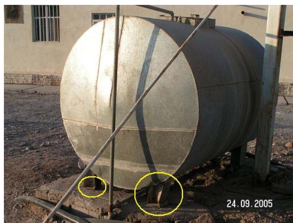
Photo 20- Buckling of feet of the water tank
