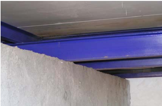
Photo 17- Operation room, bottom view
