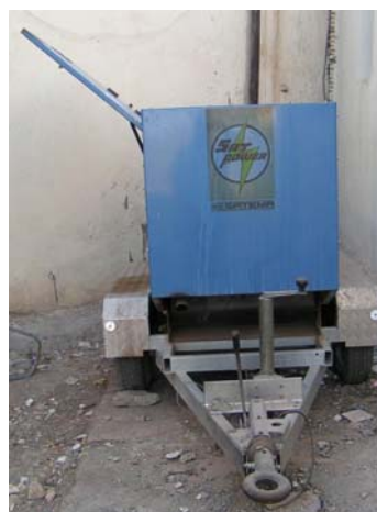
Photo 13- Electric power generator, Aflatoonian Hospital
