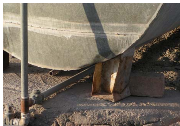
Photo 21- Buckling of feet of the water tank
