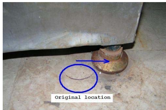
Photo 12- Displacement of a sterilizer, Aflatoonian Hospital
