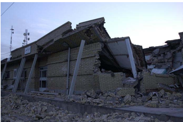
Photo 5 – Total collapse of Imam Khomeini Hospital, 2004
