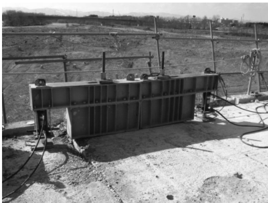
(1) 床版はく離梁
