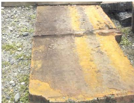
(c) 支圧板の摩耗
